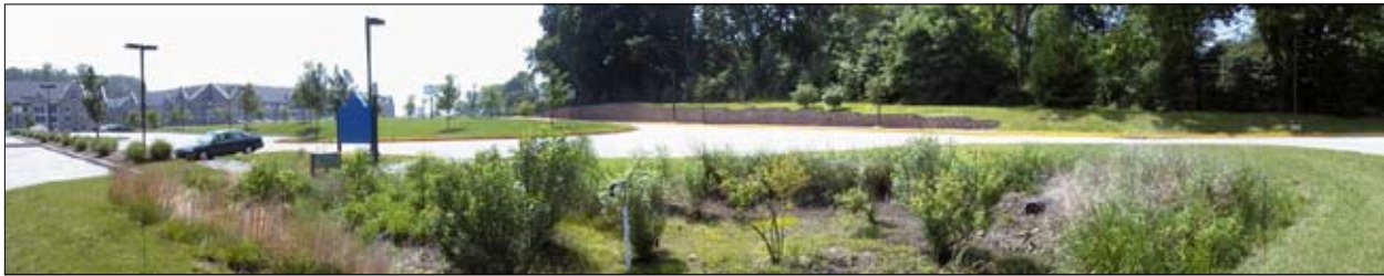
This traffic island has a “bioinfiltration” system to capture water. Photo courtesy Villanova Urban Stormwater Partnership.
