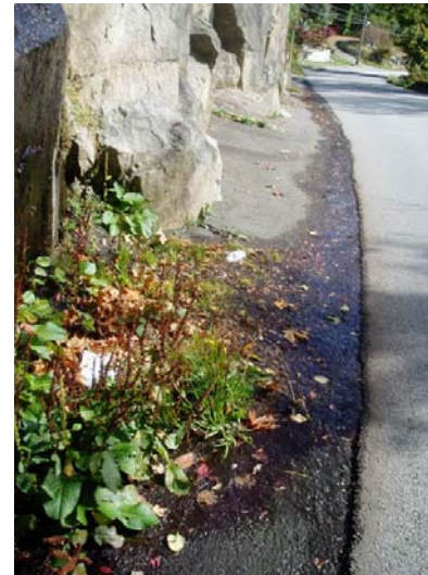
Seepage outflows onto Marine Drive are evident along the #4681 frontage, even during a summer drought.
