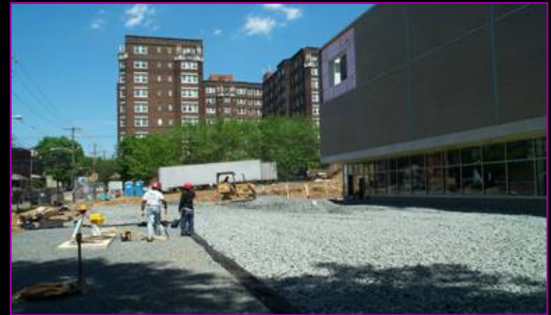
Recharge Bed under Porous Pavement Play Yard (Penn Alexander Elementary School, Philadelphia)
