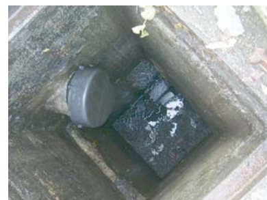
Vortex restrictor installed in a catch basin
