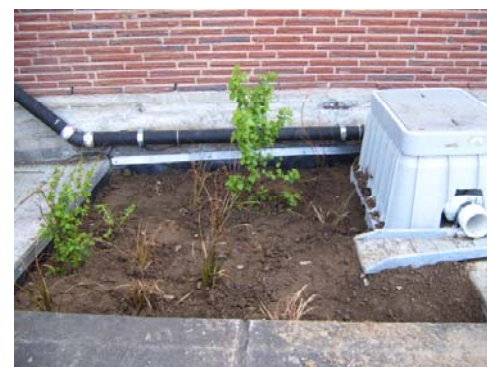
George Middle School Planter and monitoring equipment
