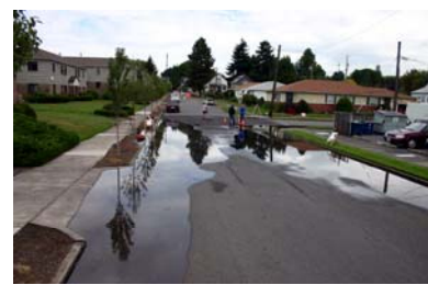
Street ponding during test at SE 41 st & Alder
