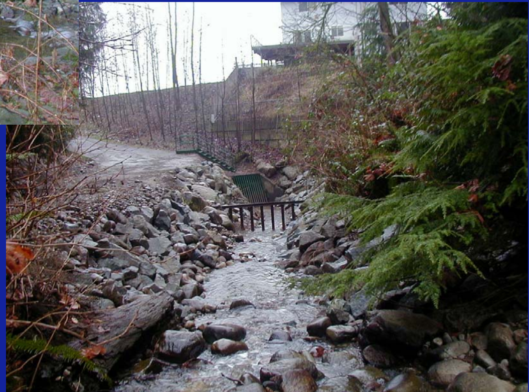
Culvert vulnerable to blockage
