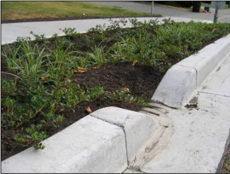
After planting; shows excess soil and incorrect grading
