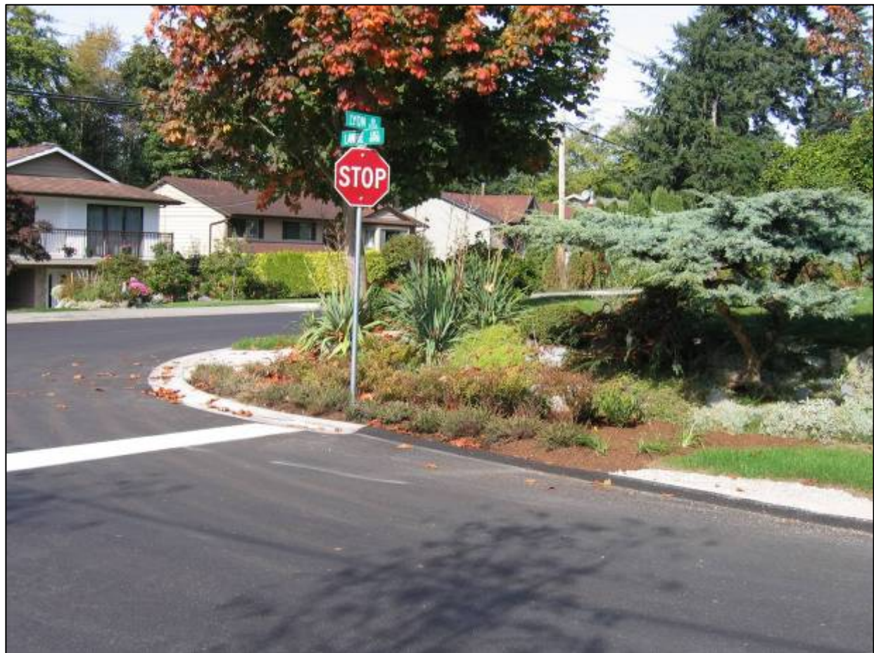
After construction (October 2006). Grass swale drains to rain garden. Overflow drain is behind the stop sign. Existing garden behind construction area was retained.
