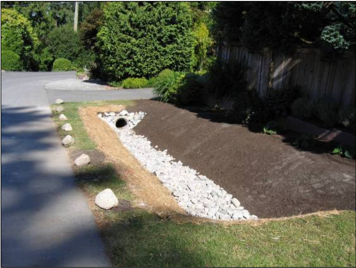
Construction complete (June 2006); temporary mesh installed on road side of ditch to minimize erosion until plants are installed
