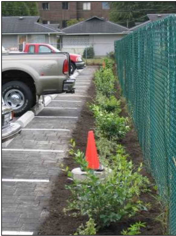
Planting bed for stormwater collection (west side)
