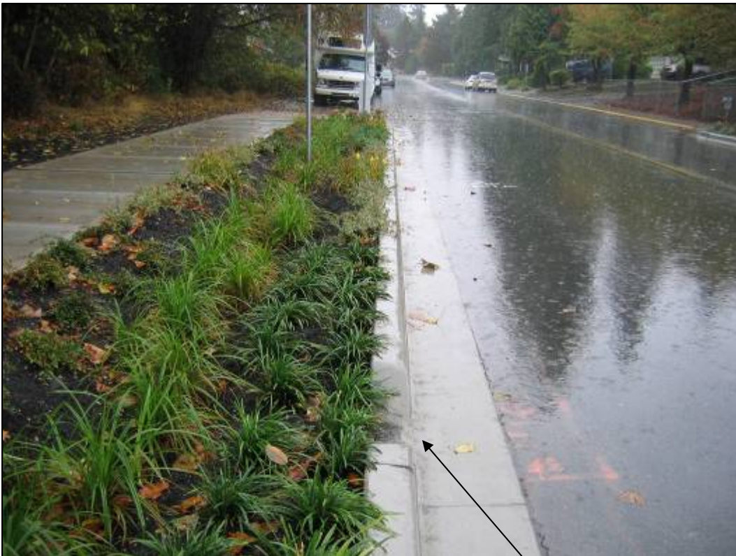
North side during heavy rainfall event (September 2005); runoff entering from the curb cut was absorbed by the drain rock within 50cm of entering the swale
