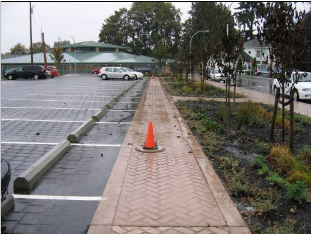
Completed project after heavy rainfall event; note pooling of water between asphalt parking lot and concrete walkway, and within the planting area
