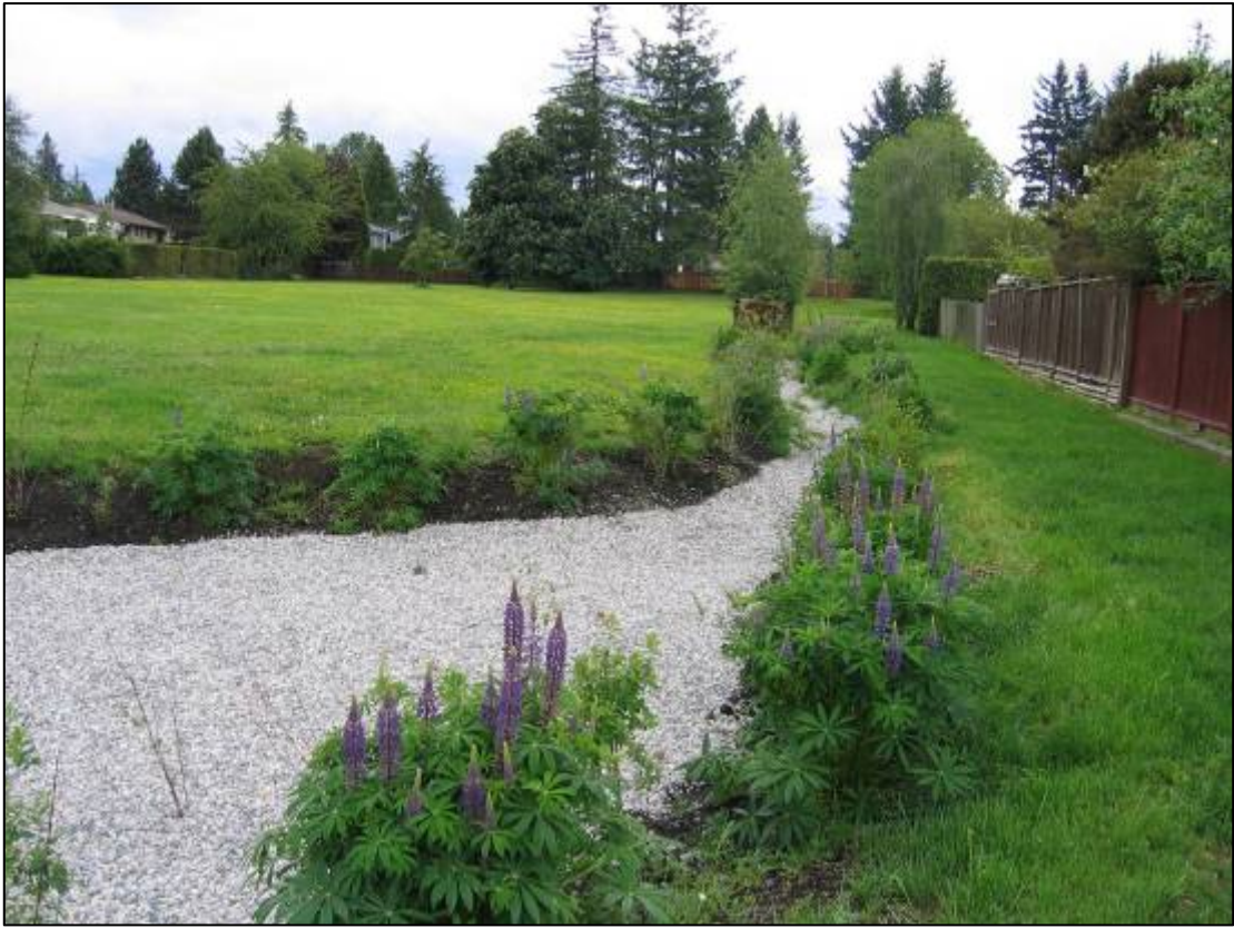
Placement of rock in swale to prevent erosion and standing water (July 2006)
