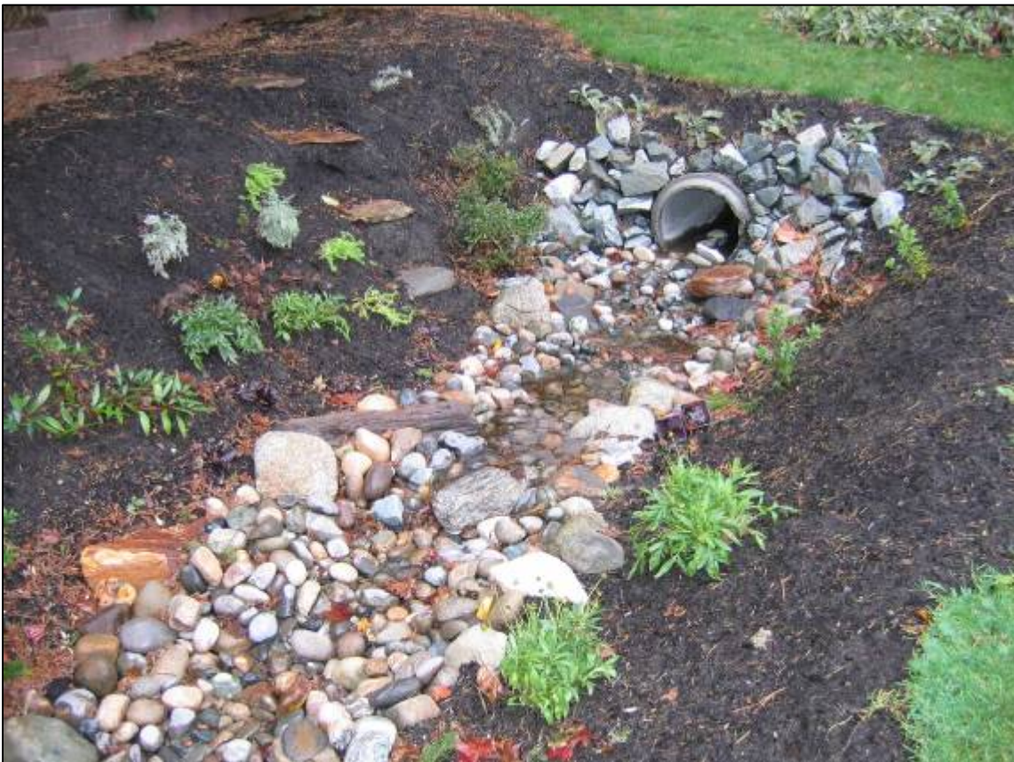
During heavy rainfall event (November 2006)
