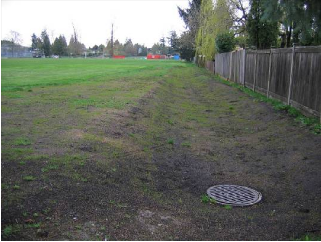
Swale after re-grading to make shallower for sports field users; planted with grass (April 2006)
