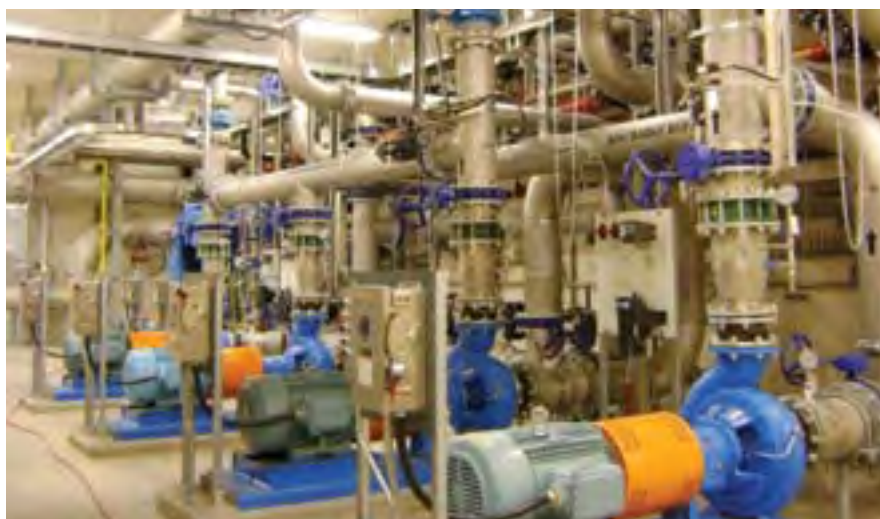
Process pipe gallery and primary filtration pumps.
