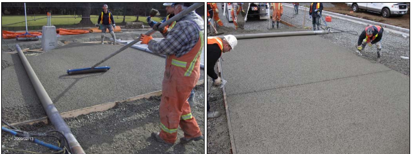
Fig. 4.3 – (a) Cross roller to improve surface finish (b) Hand float and an edging tool used to prevent ravelling of the edges
