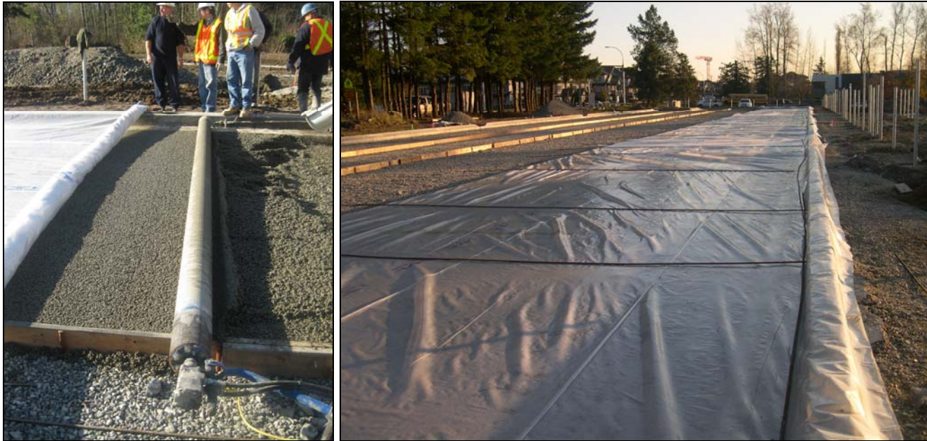
Fig. 4.4 – Curing with heavy plastic sheeting began immediately and continued for a period of 7-days.
