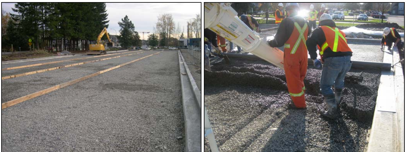
Fig. 4.1 – Preparation of the base course material. Truck ruts are raked out prior to pervious concrete placement.
