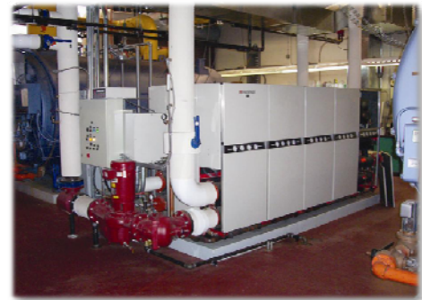
Okanagan College Heat Pumps
